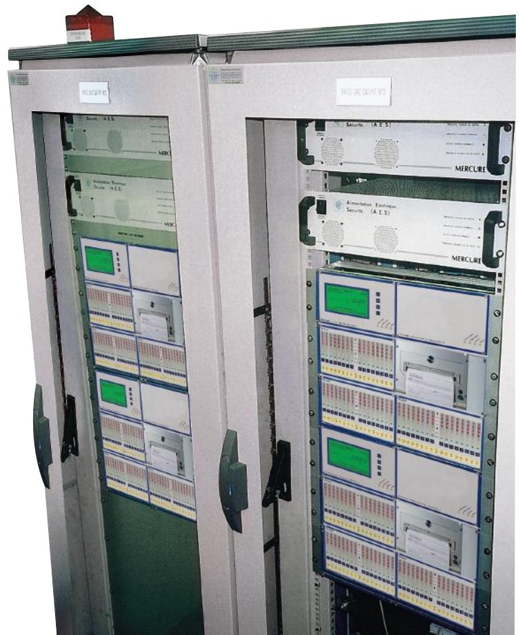
Example of installation with 256 detectors
